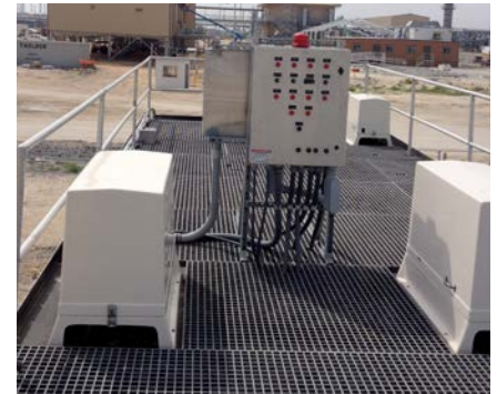
Electrical Control Console
