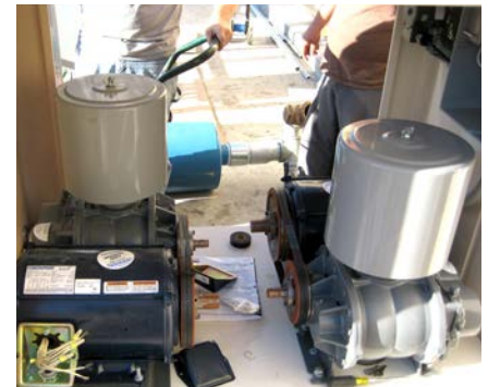
Air Blower Unit
